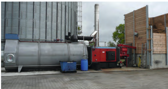
Indirect STELA air heater with Bioflamm combustion plant
